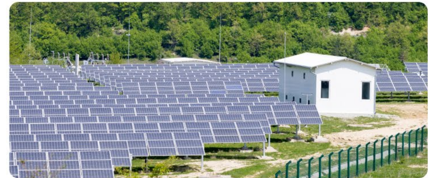
Solar power plant
